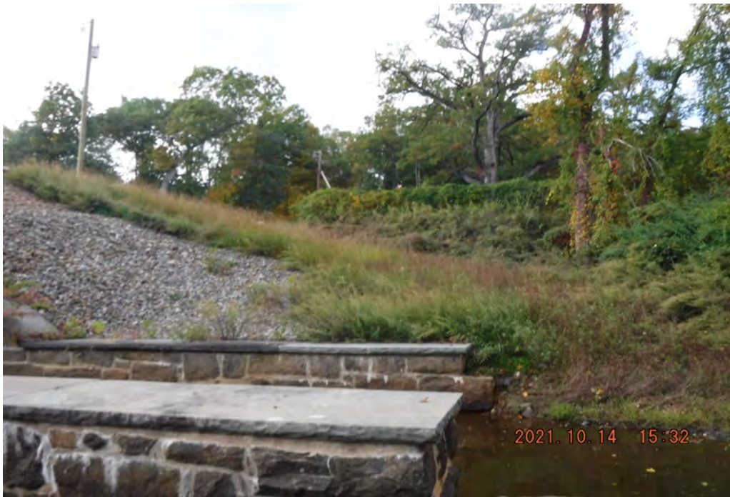
Photo 6 Dam ID# 196-0361 Lower Wee-wah Lake Dam 10/14/2021 Left downstream slope View looking left from right side of spillway
