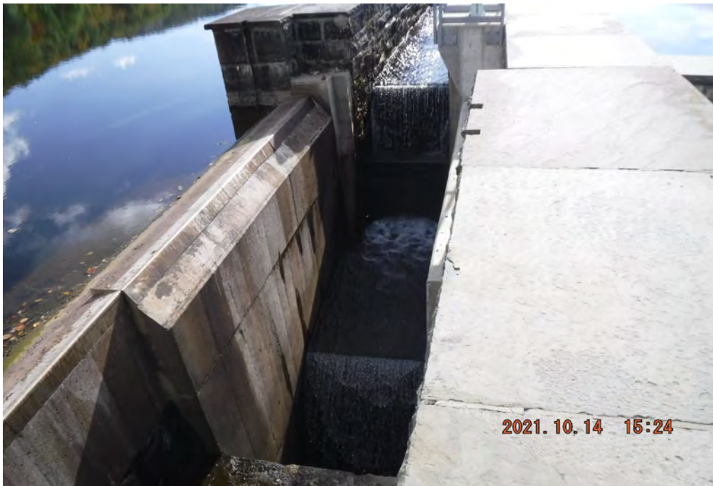
Photo 12 Dam ID# 196-0361 Lower Wee-wah Lake Dam 10/14/2021 Spillway outlet channel View looking upstream from left side of channel
