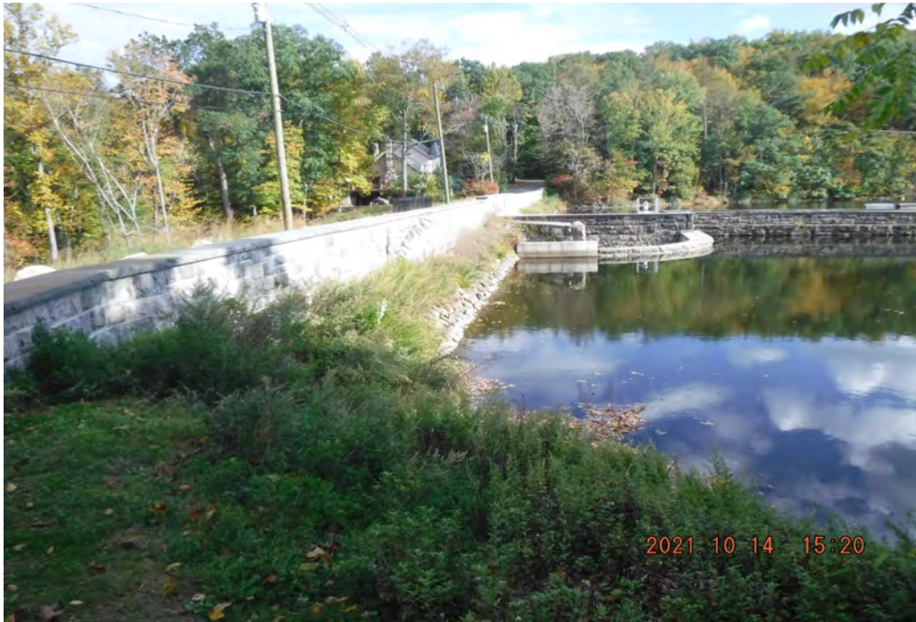
Photo 1 Dam ID# 196-0361 Lower Wee-wah Lake Dam 10/14/2021 Left upstream slope View looking right from left end of dam
