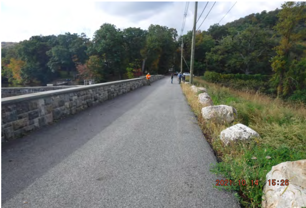
Photo 4 Dam ID# 196-0361 Lower Wee-wah Lake Dam 10/14/2021 Dam crest View looking left from right end of dam
