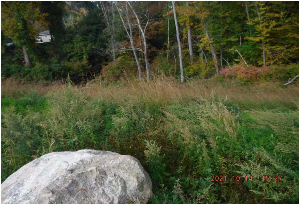
Photo 5 Dam ID# 196-0361 Lower Wee-wah Lake Dam 10/14/2021 Right downstream slope View looking downstream from crest
