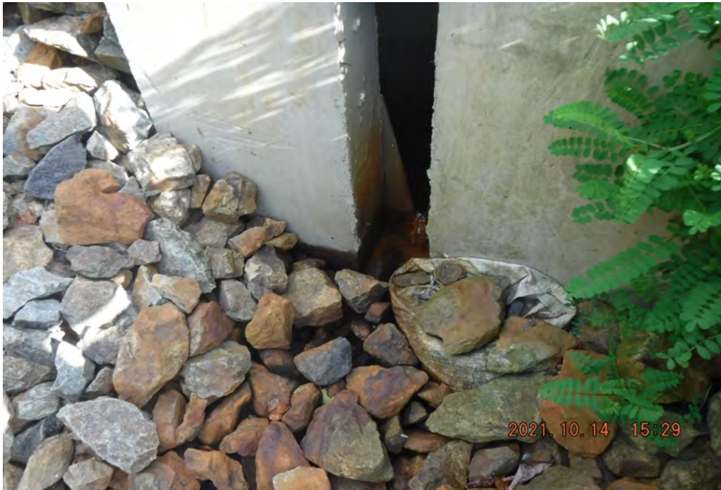
Photo 7 Dam ID# 196-0361 Lower Wee-wah Lake Dam 10/14/2021 Weir box for right downstream toe drain
