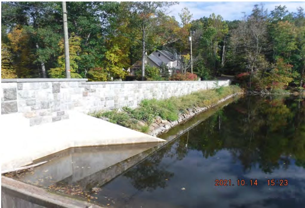
Photo 2 Dam ID# 196-0361 Lower Wee-wah Lake Dam 10/14/2021 Right upstream slope View looking right from spillway channel
