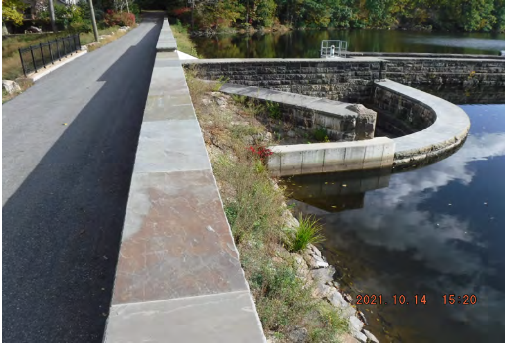
Photo 15 Dam ID# 196-0361 Lower Wee-wah Lake Dam 10/14/2021 Auxiliary spillway View looking right from the left side
