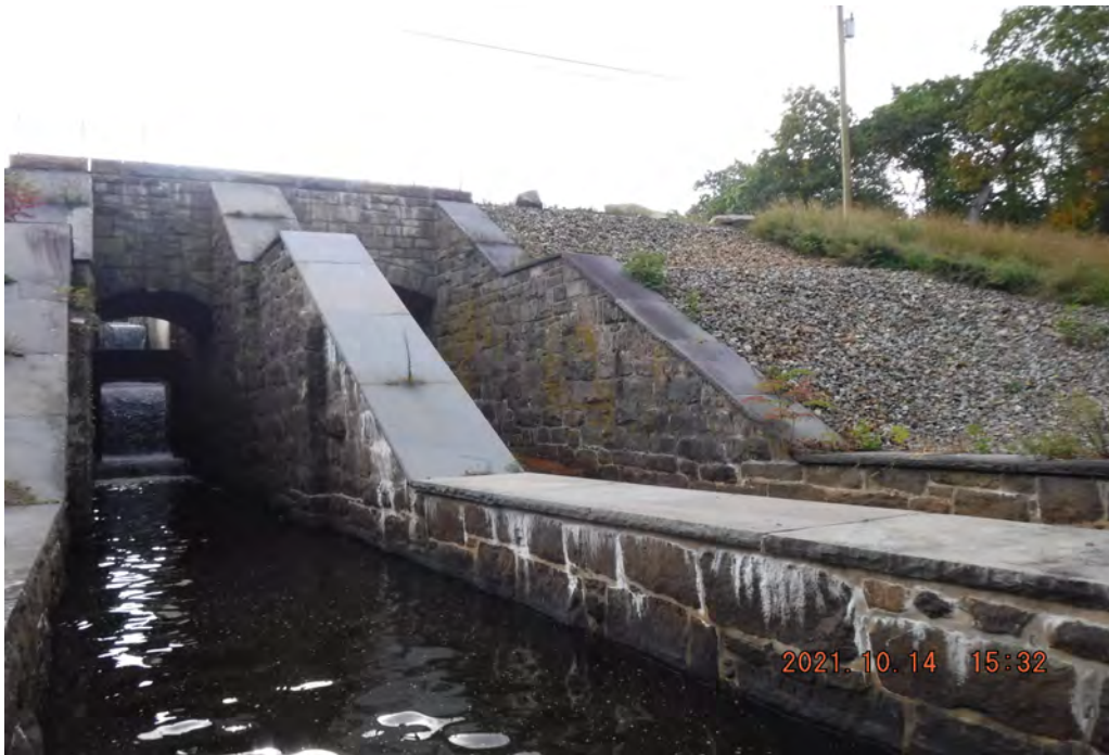
Photo 13 Dam ID# 196-0361 Lower Wee-wah Lake Dam 10/14/2021 Spillway outlets View looking upstream from downstream right side
