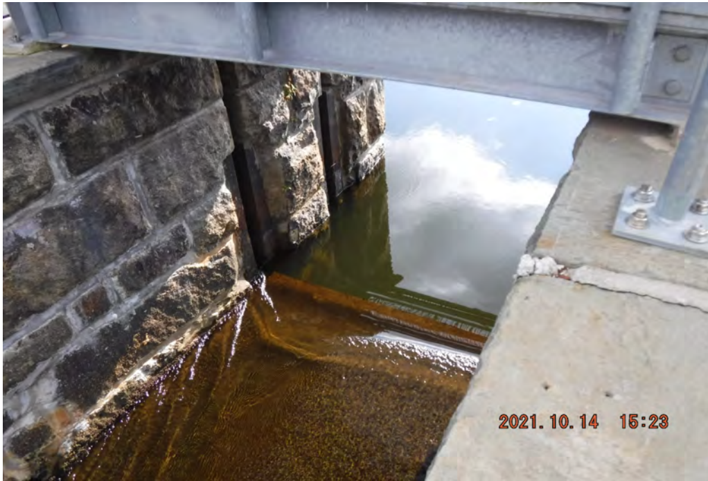
Photo 9 Dam ID# 196-0361 Lower Wee-wah Lake Dam 10/14/2021 Primary spillway inlet with stop logs View looking upstream from left side
