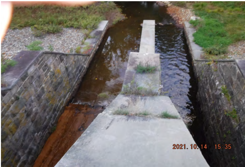
Photo 14 Dam ID# 196-0361 Lower Wee-wah Lake Dam 10/14/2021 Downstream spillway outlets View looking downstream from dam crest
