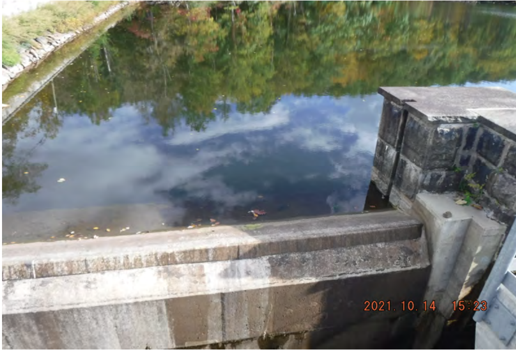
Photo 11 Dam ID# 196-0361 Lower Wee-wah Lake Dam 10/14/2021 Secondary spillway on right side of spillway channel View looking right from left side
