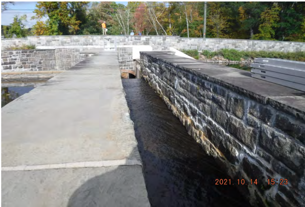
Photo 10 Dam ID# 196-0361 Lower Wee-wah Lake Dam 10/14/2021 Spillway channel View looking downstream from spillway inlet
