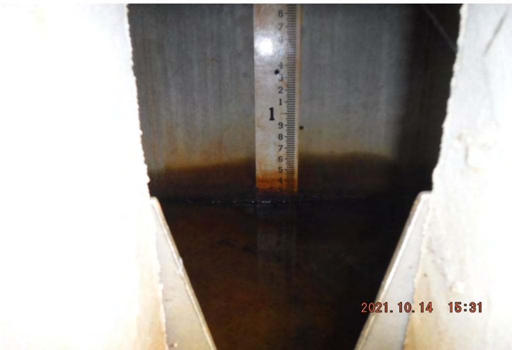
Photo 8 Dam ID# 196-0361 Lower Wee-wah Lake Dam 10/14/2021 Inside weir box for right downstream toe drain Gauge reads 2-inches +/-
