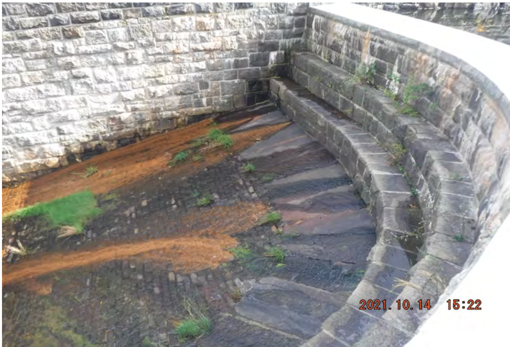
Photo 16 Dam ID# 196-0361 Lower Wee-wah Lake Dam 10/14/2021 Downstream face of auxiliary spillway View looking upstream to the right from dam crest Note: seepage through spillway floor
