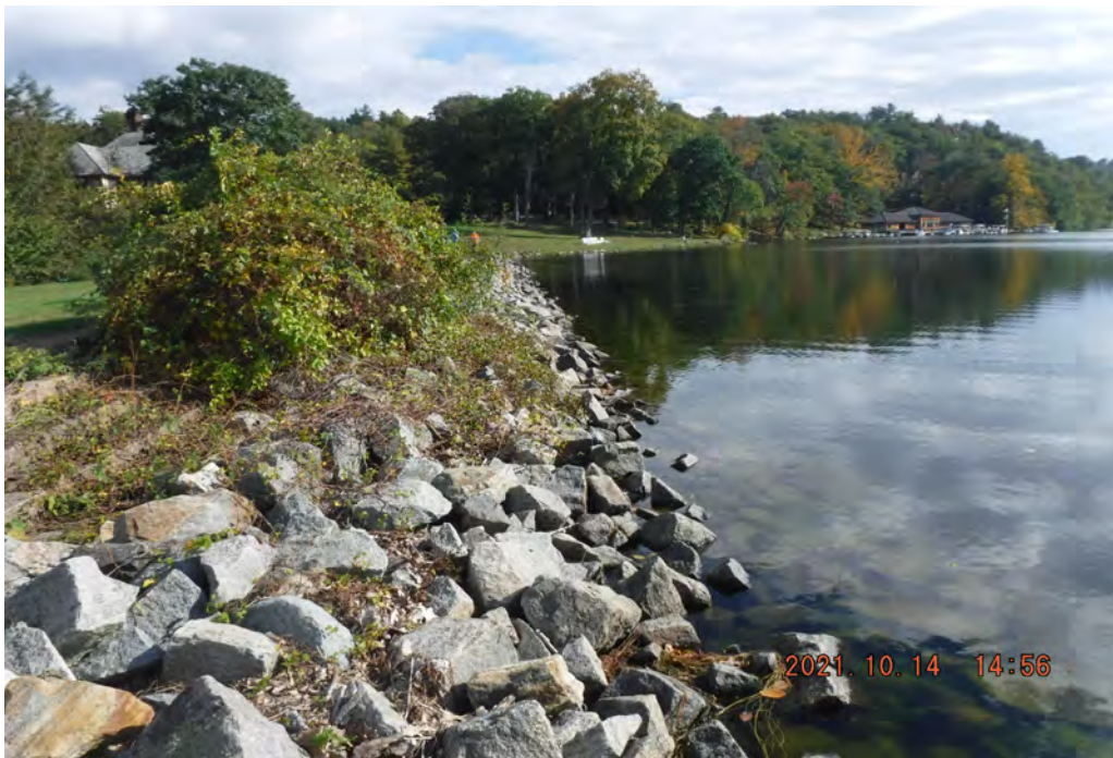
Photo 4 Dam ID# 196-0354 Tuxedo Lake Dam 10/14/2021 Upstream slope around concrete steps View looking right from left side
