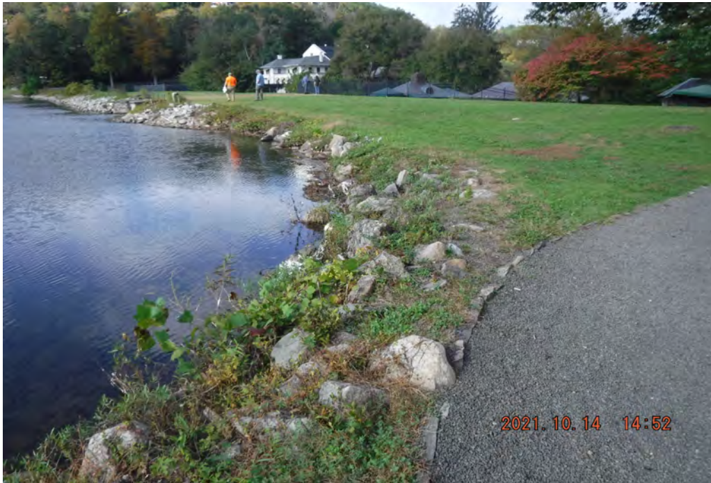
Photo 1 Dam ID# 196-0354 Tuxedo Lake Dam 10/14/2021 Right end of upstream slope View looking left from right end of dam
