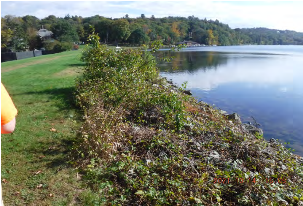
Photo 3 Dam ID# 196-0354 Tuxedo Lake Dam 10/14/2021 Upstream slope View looking right from left end of dam
