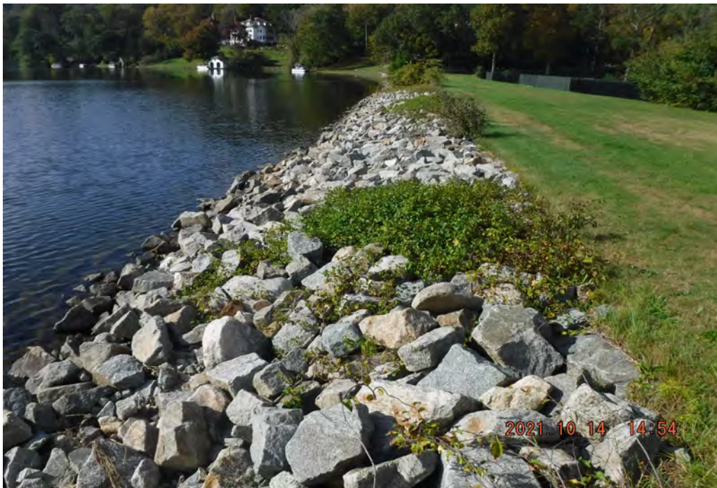
Photo 2 Dam ID# 196-0354 Tuxedo Lake Dam 10/14/2021 Left upstream slope View looking left from service spillway
