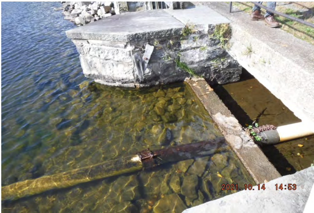
Photo 8 Dam ID# 196-0354 Tuxedo Lake Dam 10/14/2021 Right spillway View looking left from right side of spillway
