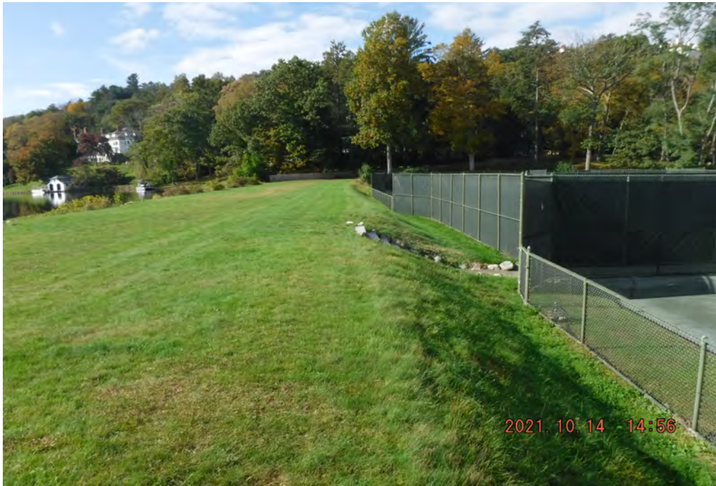
Photo 7 Dam ID# 196-0354 Tuxedo Lake Dam 10/14/2021 Left downstream slope View looking left from service spillway
