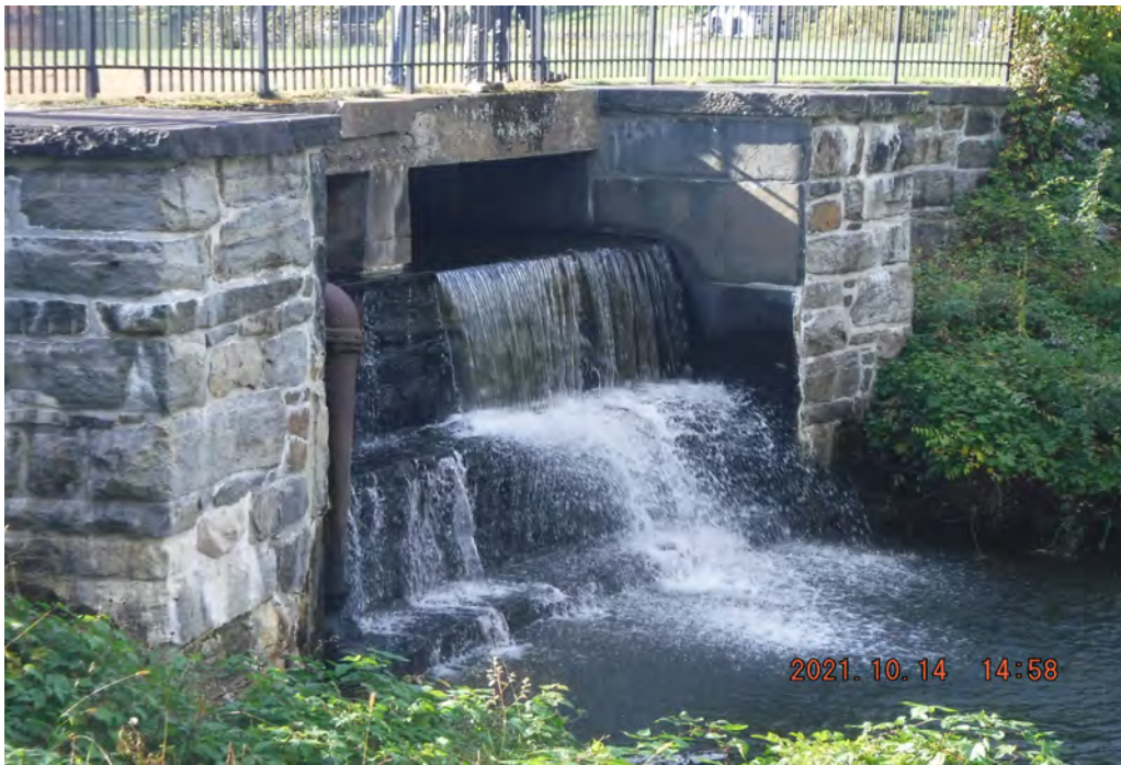
Photo 10 Dam ID# 196-0354 Tuxedo Lake Dam 10/14/2021 Service spillway downstream outlet View looking upstream to the left from right side of channel
