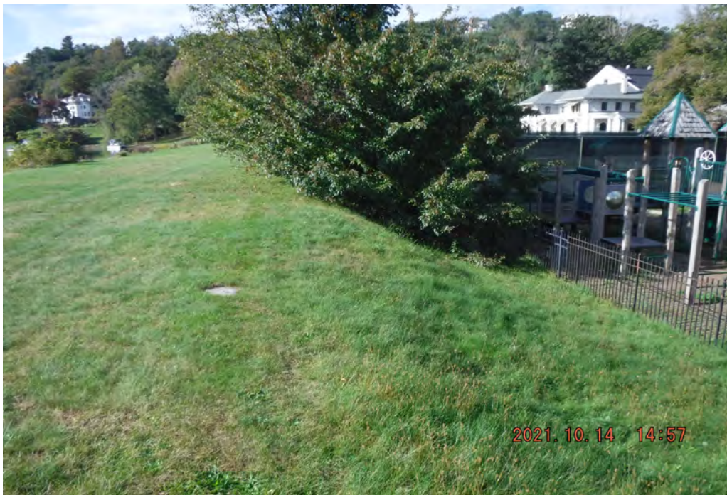
Photo 6 Dam ID# 196-0354 Tuxedo Lake Dam 10/14/2021 Downstream slope View looking left from service spillway
