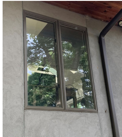
WINDOWS ANDERSEN WINDOWS A-SERIES TERRATONE COLOR EXISTING TO REMAIN AND/OR NEW TO MATCH
