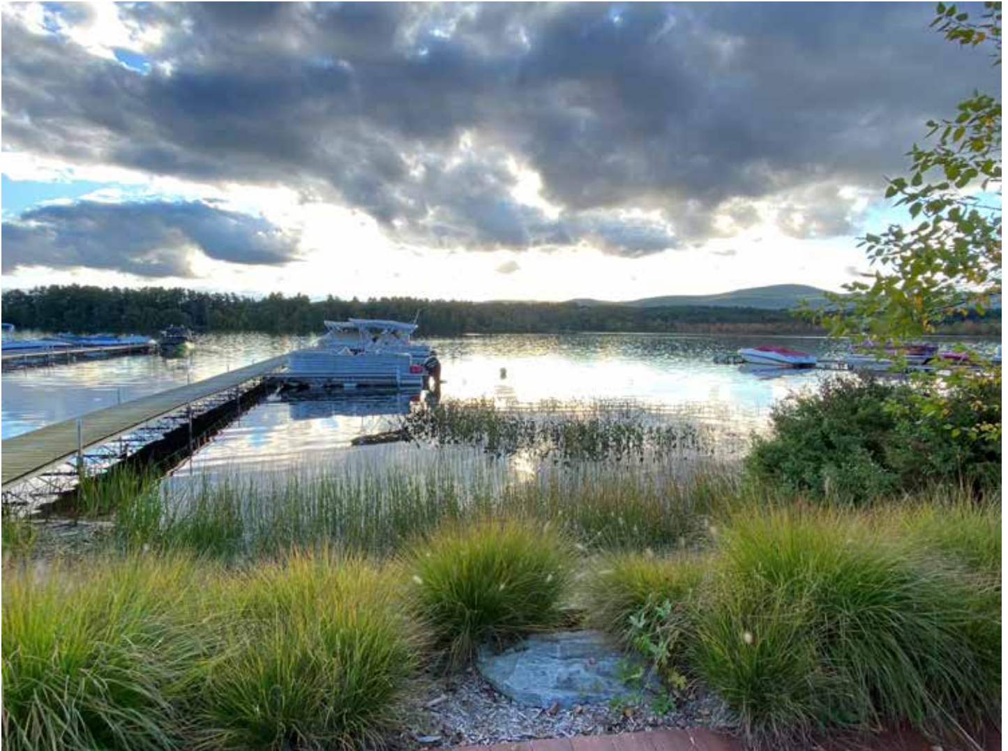
MKM planned and built a seasonal dock. Native grasses are planted to stabilize the shoreline.
