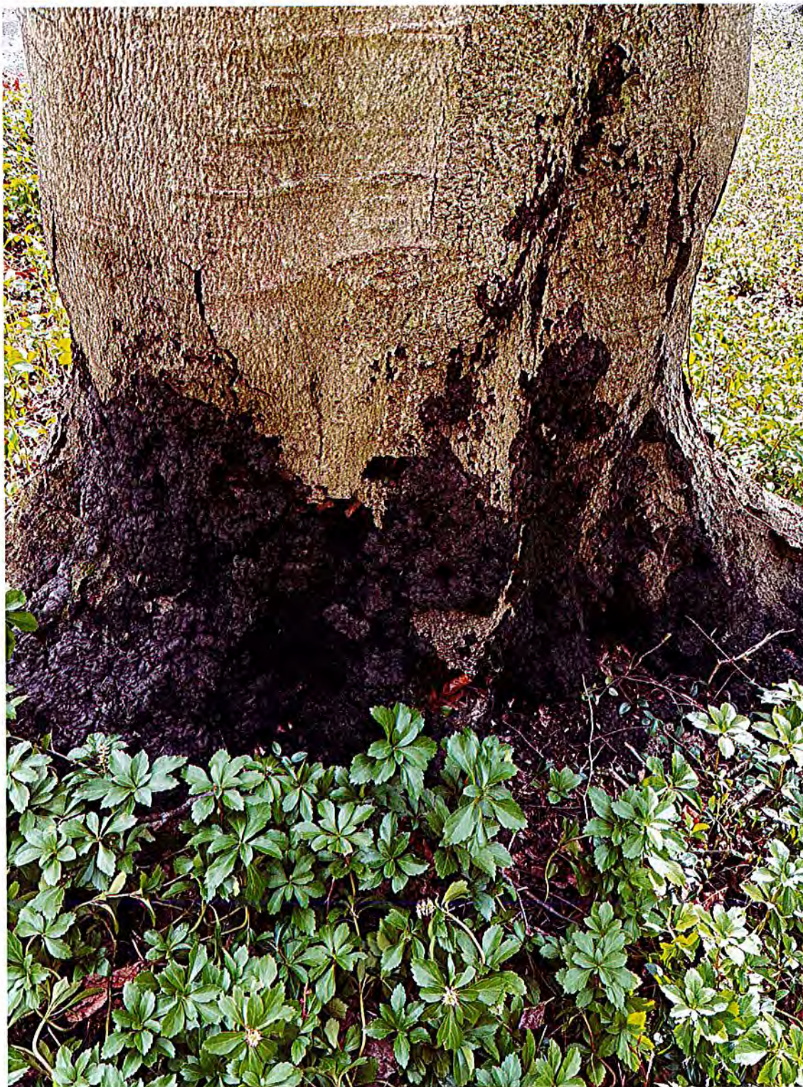
American beech #9 recommended for removal because of decay and suspected fungi at root flare.
